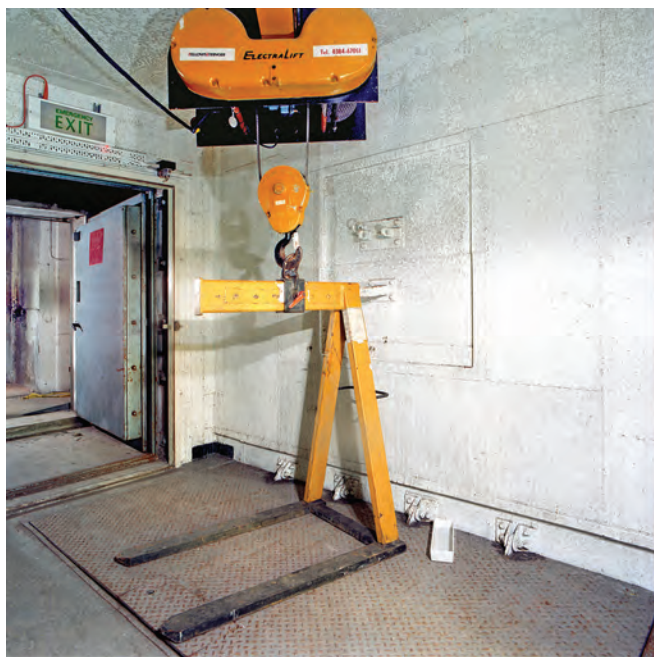
Hydraulically operated trap door and hoist near the emergency exit. This allowed equipment to be lowered to the levels below. Photo Nick Catford
